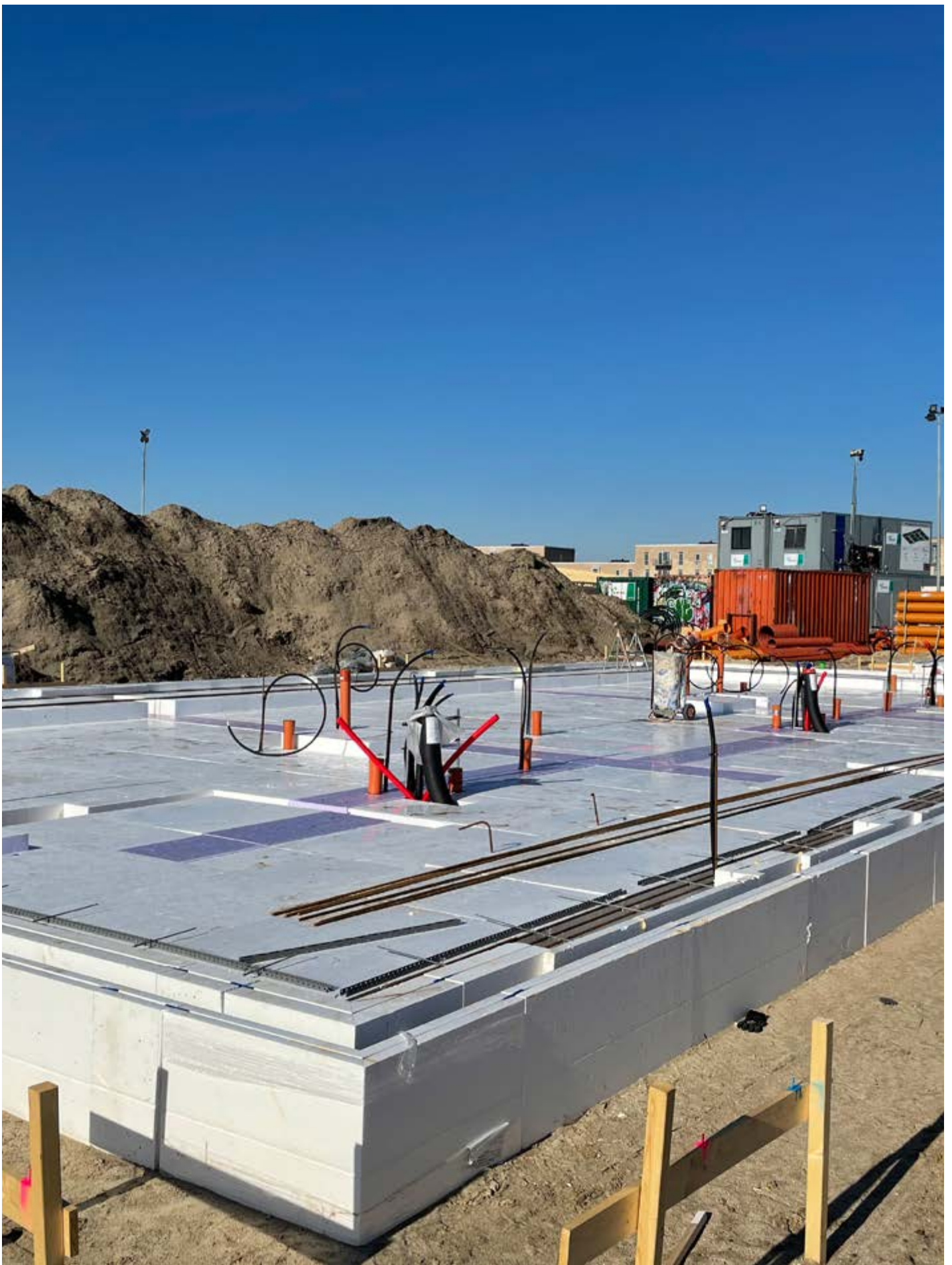
The contractor HP Byg used the foundation system in the building of 43 townhouses in Aalborg, Denmark.
