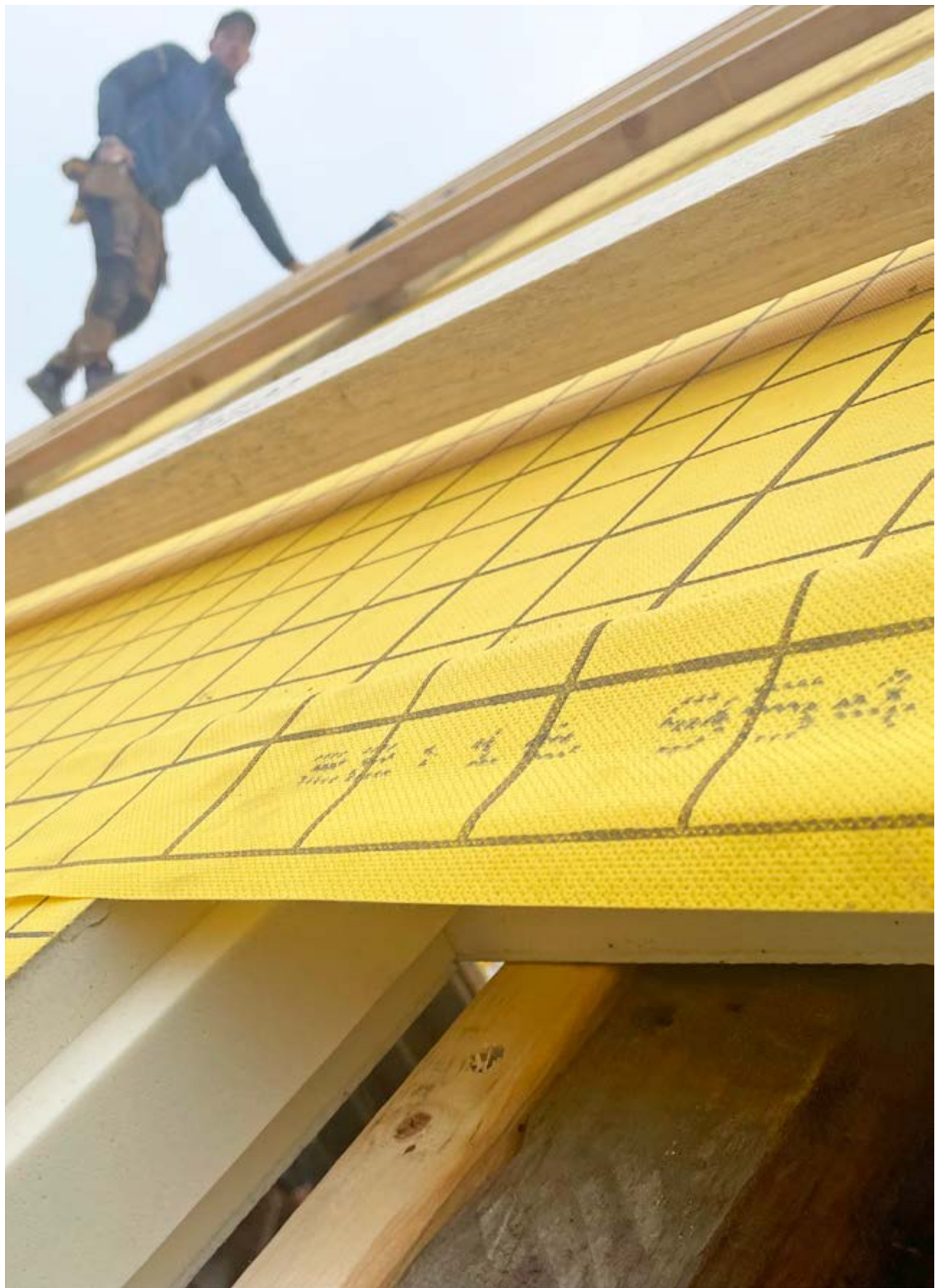
The architectural firm Møller Nielsens Tegnesteue, based in Struer, designed the new roof for Struer Fri- og Fag-skole, which was installed by Rosenberg Madsen. The architect opted for a polyisocyanurate insulation to maximize space and maintain the roof's aesthetic appeal.
