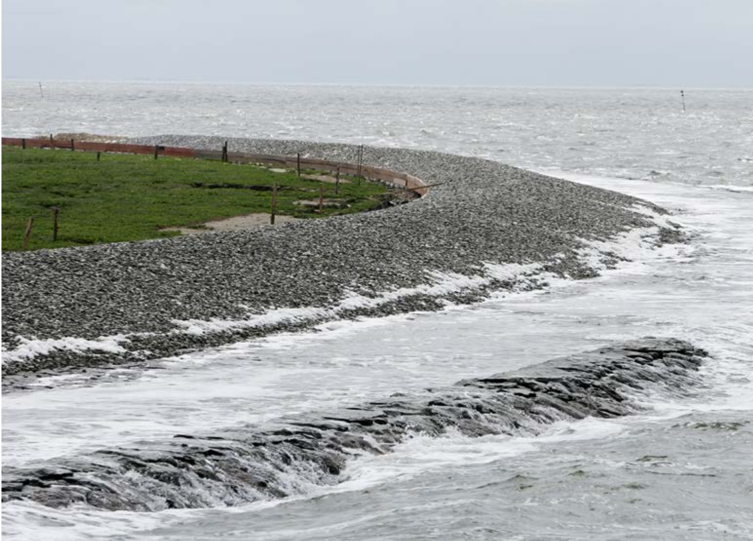
Coastal protection with minimal material consumption and space for flora and fauna. Sources: Heijmans & BASF
