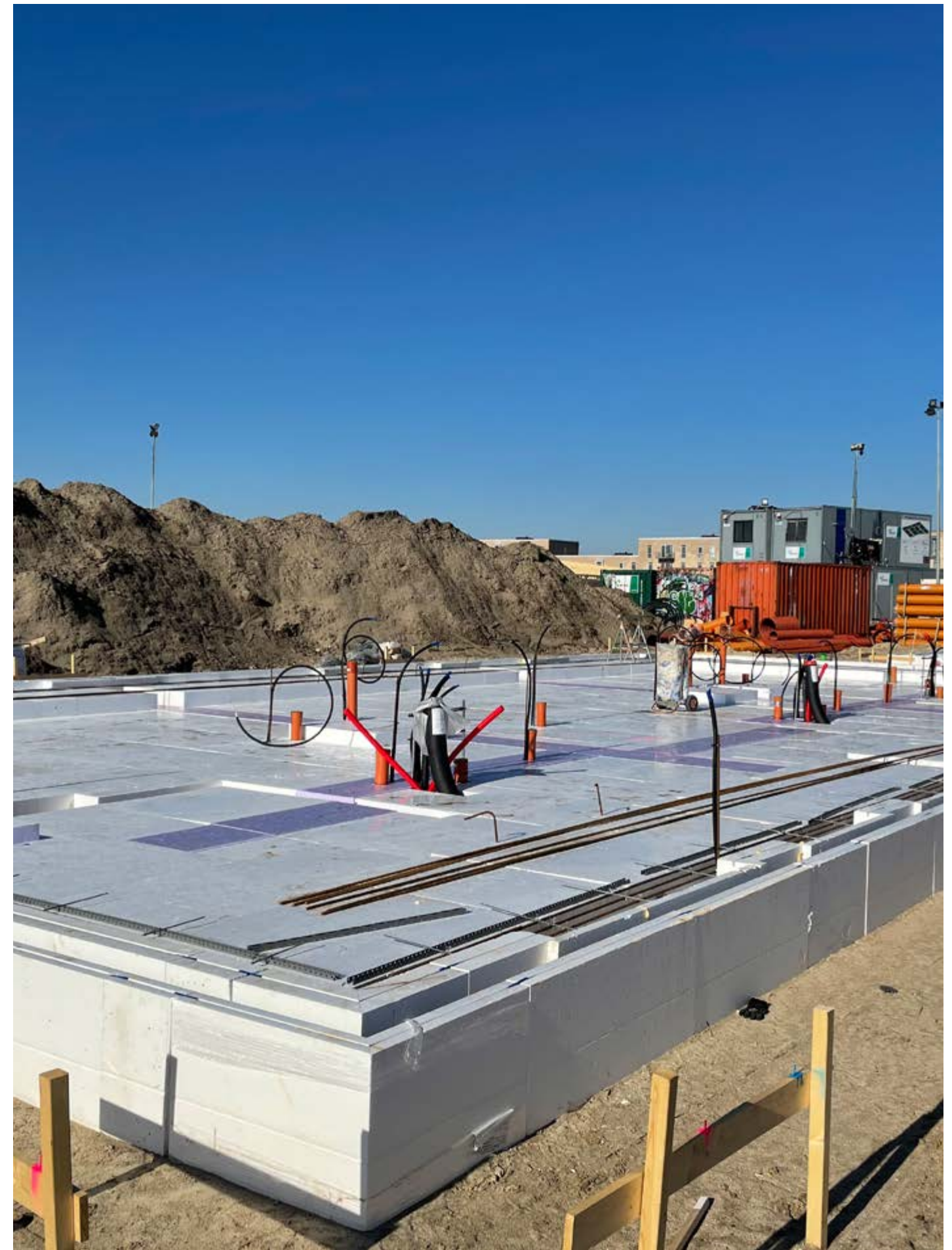
The contractor HP Byg used the foundation system in the building of 43 townhouses in Aalborg, Denmark.
